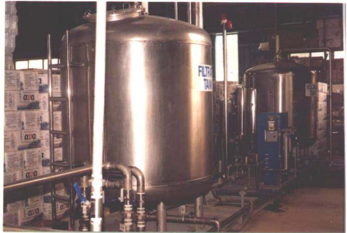
Water Treatment System
