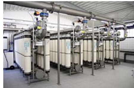
Drinking water treatment 300 m 3 /h using ultrafiltration in Grundmühle waterworks (Germany)
